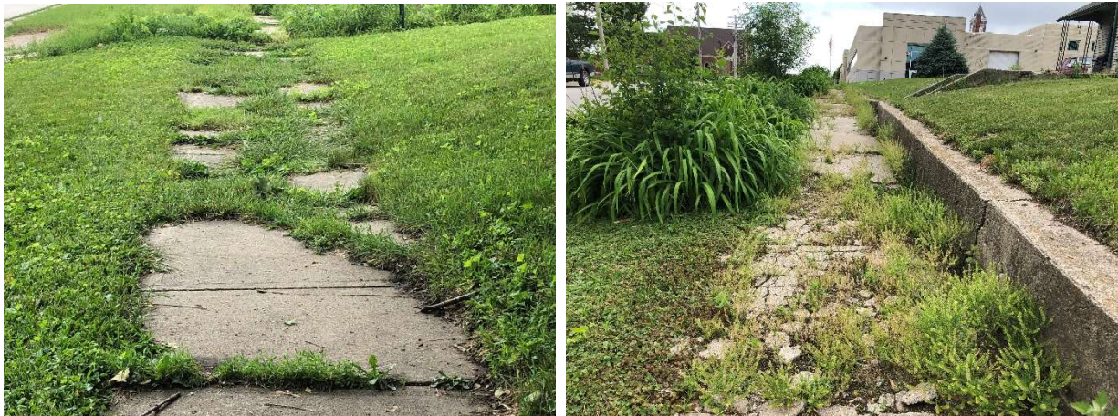
Privately owned sidewalk segments in need of repair in a town of around 2,500 population in RPA 6 region.
